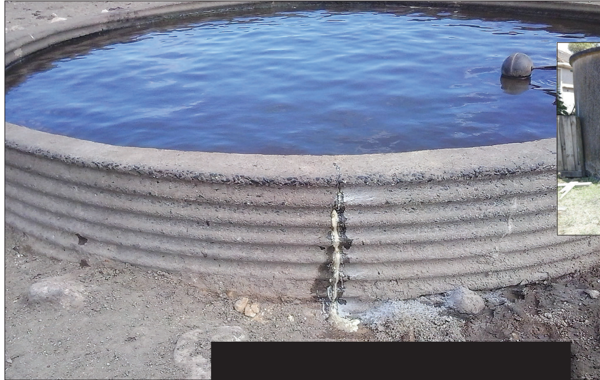
A leaking concrete water tank will prove costly over time.
